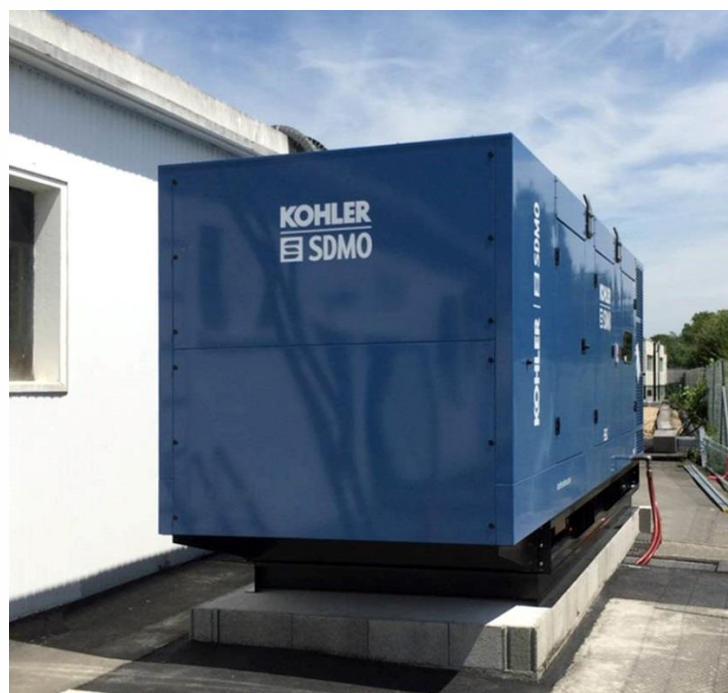
Pic. 2: The KD900 generating set in enclosure version at the Ancenis water treatment plant.
