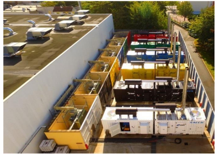
Pic. 2. The six new generating sets have been connected to the first installation and each has a defined colour code.
